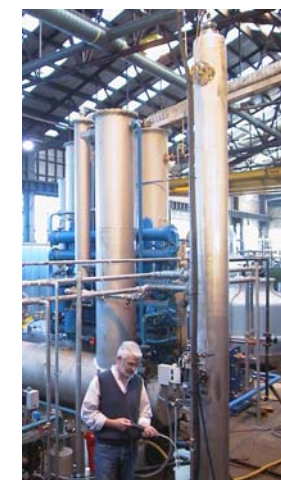
High Pressure Purifier
